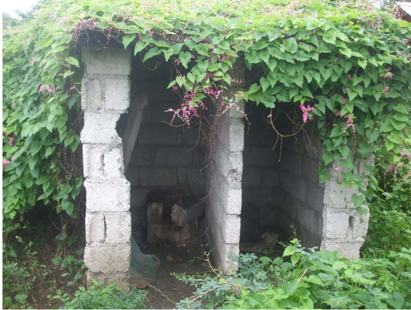
FIGURE 8: EXEMPLE DE TOILETTE COLLECTIVE NON ENTRETENUE
