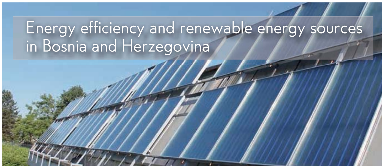
Thermal solar collectors at Sports and Culture Centre in Tuzla, Bosnia and Herzegovina
